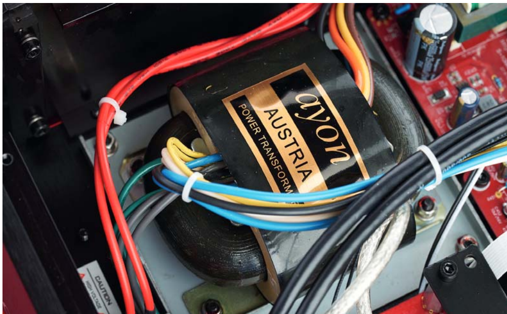
The big R-Core transformer
